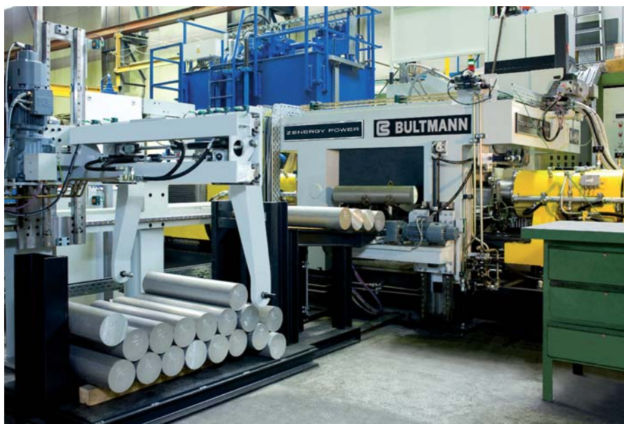
Magnetic billet heater operating at Weseralu aluminum profile extrusion plant
